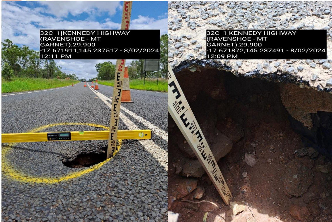
Photos 5 and 6. Sink hole near centreline
