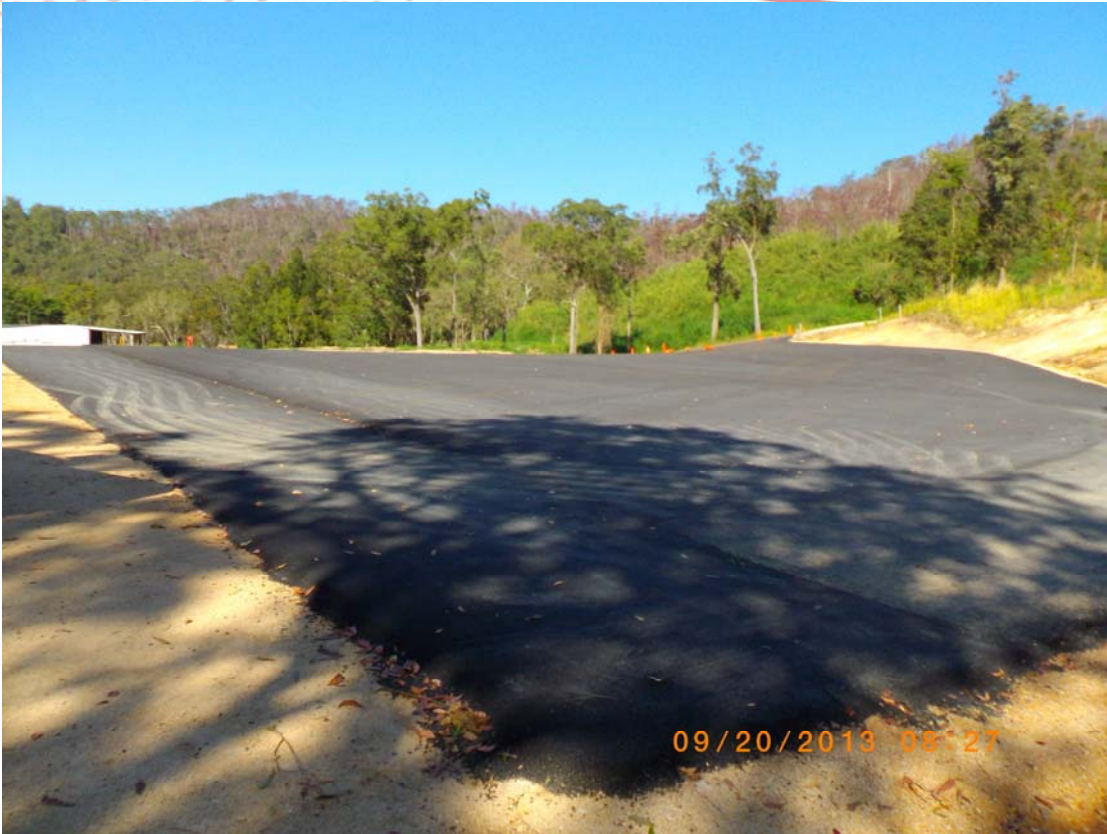
Figure 4: Atherton waste transfer station buy back shop foundation
